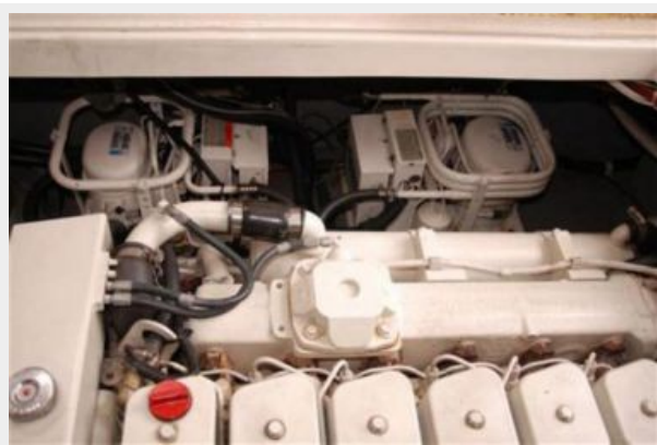
AC's Installed in Engine Room
