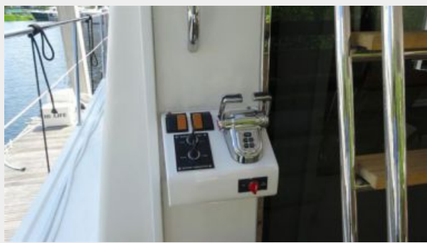
Aft Deck control station
