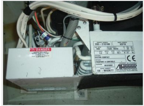
Air Conditioning unit
