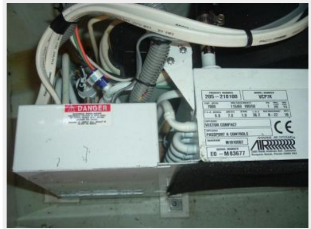
Air Conditioning unit
