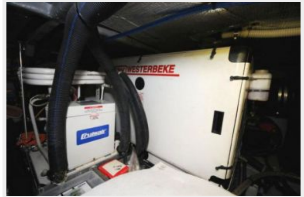
Generator with Sound Shield
