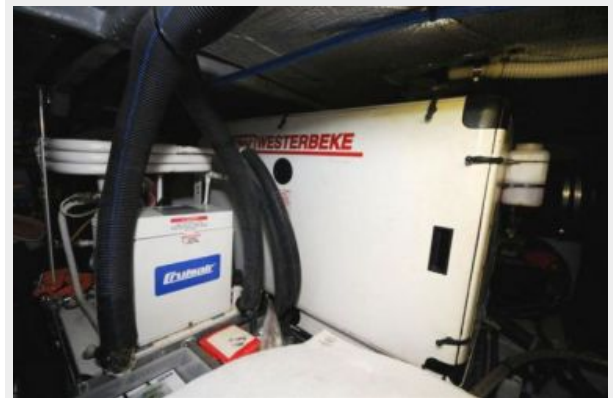
Generator with Sound Shield
