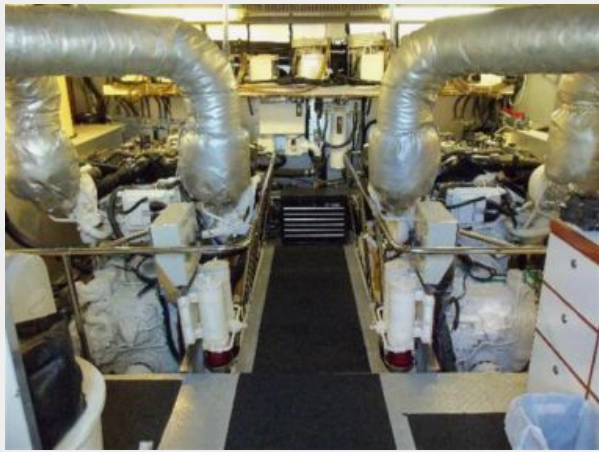
Engine Room Looking Forward
