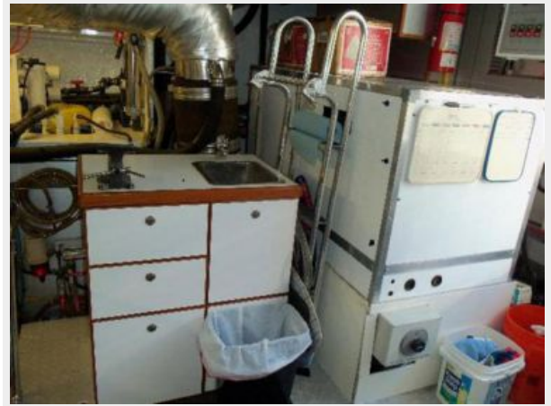
Starboard Generator & Workbench
