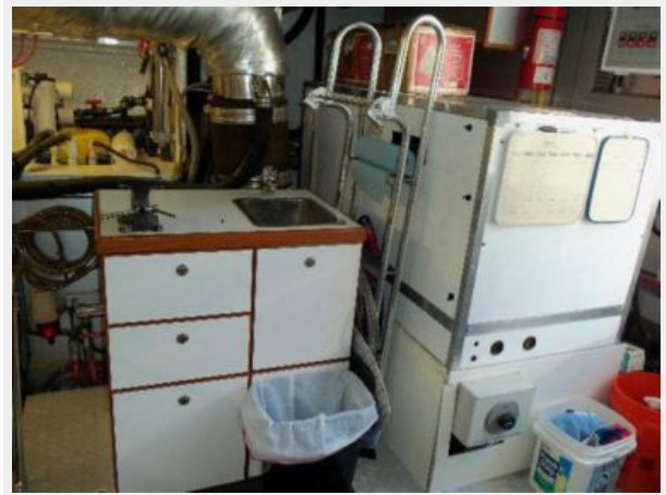
Starboard Generator & Workbench
