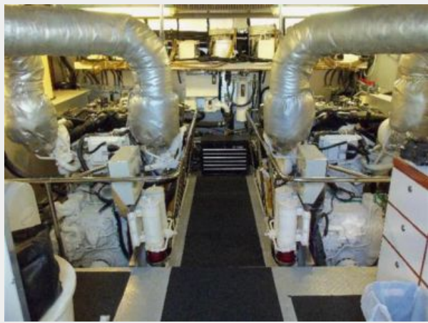
Engine Room Looking Forward
