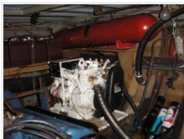
Onan Genset with Fire Suppression System
