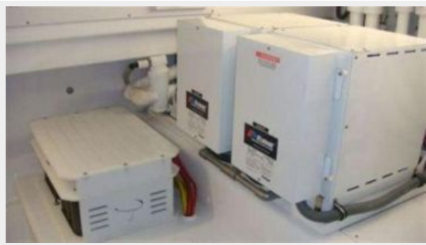
Chilled Water A/C
