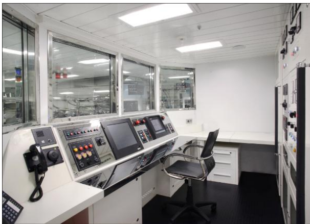
Engineer's control room
